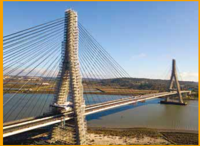
The 100m-high pylons of the Gadiana International Bridge were covered with ULMA's BRIO Modular Scaffolding to facilitate the repair of suspension cables (image courtesy ULMA)
